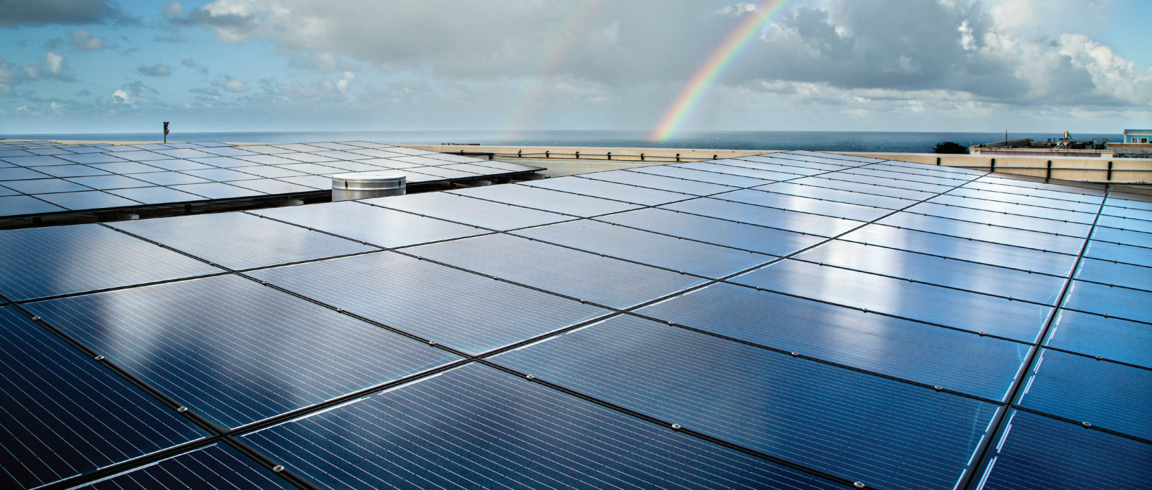
Solar panels at the rooftop of Ballajá Infantry Barracks Building (Cuartel de Infantería de Ballajá) in Old San Juan, San Juan, P.R., on March 26, 2021. (Erika P. Rodriguez for Earthjustice)
